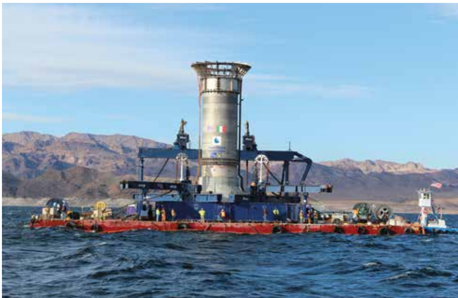
Figure 3. Third intake structure being prepared for placement in Lake Mead. Drought conditions were a significant factor in driving the construction of a new drinking water intake despite the significant cost. Photo: Southern Nevada Water Authority Engineering.
